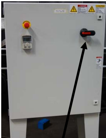
Container/Trolley Drive Breaker (Disconnect Switches)
