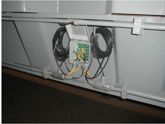
Summing box where all load cells are connected.
