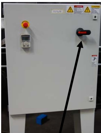
Container/Trolley Drive Breaker (Disconnect Switches)
