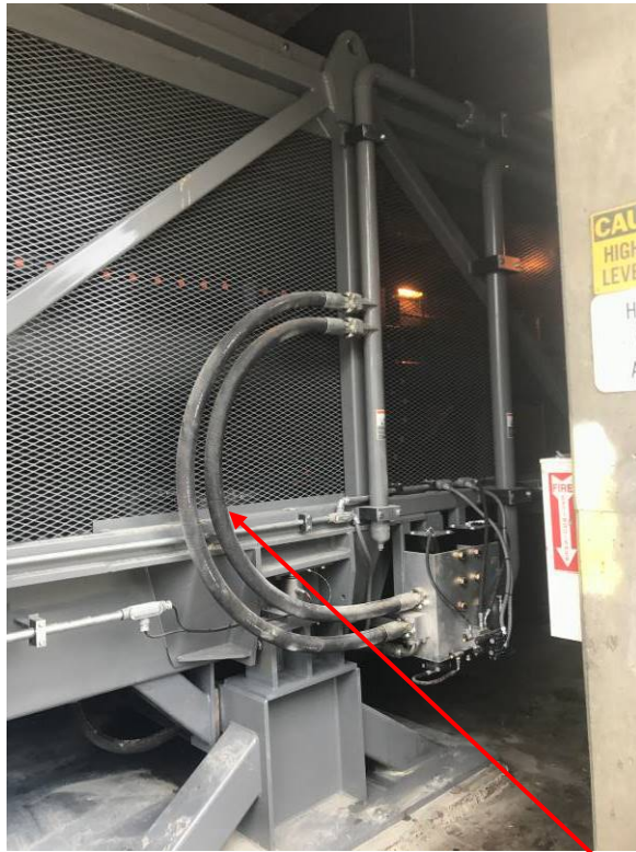
As you can see here that there are two pressure hose connections
