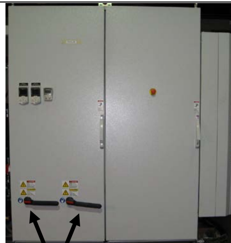
Compactor Main Power Breakers (Disconnect Switches)
