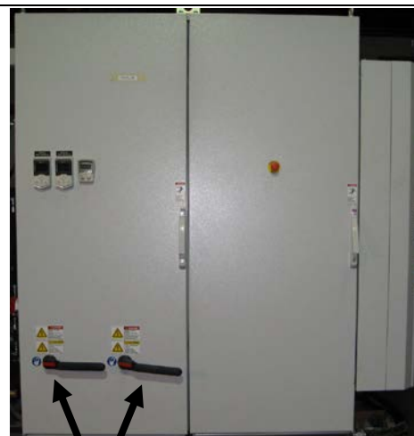
Compactor Main Power Breakers (Disconnect Switches)
