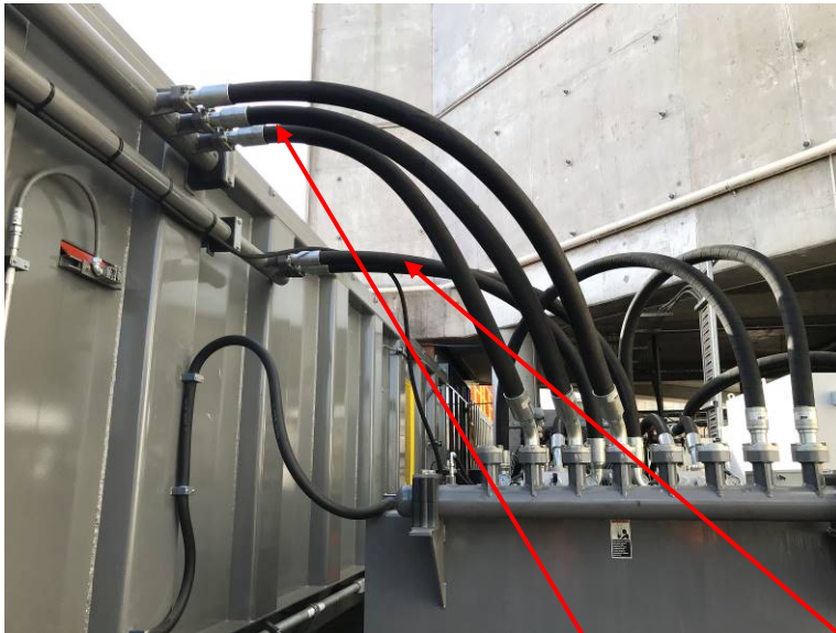
As you can see here that there are three return hoses and two pressure hoses
